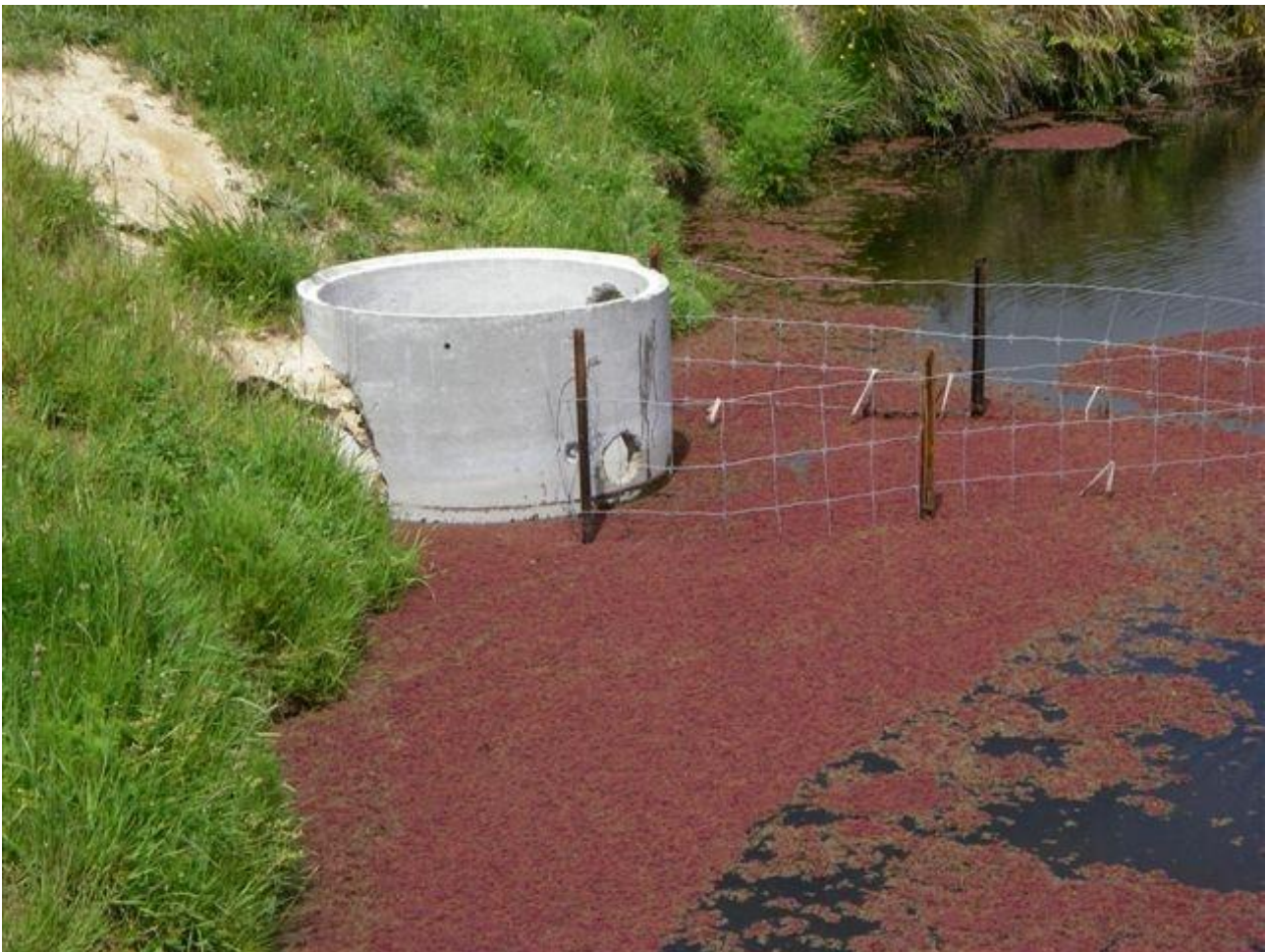
Figure 2: Adapted outlet riser, installed at the existing farm dam in the upper Ōkaro catchment. Photo supplied by John Paterson, BoPRC.
